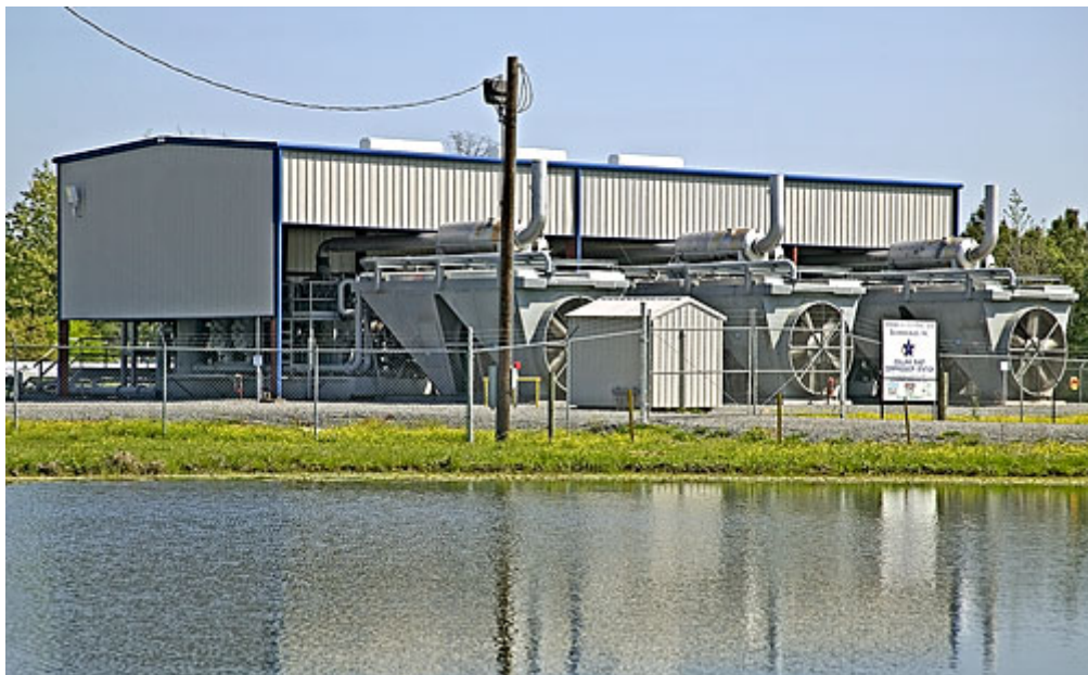
Figure 2-1. Large compressor station (American Central Gas Compressor Station; Carthage, TX).
