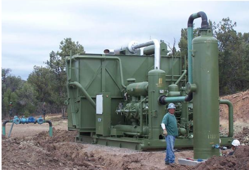
Figure 2-2. Medium size gas compressor engine installation (Evaporative Systems Inc, 2005).
