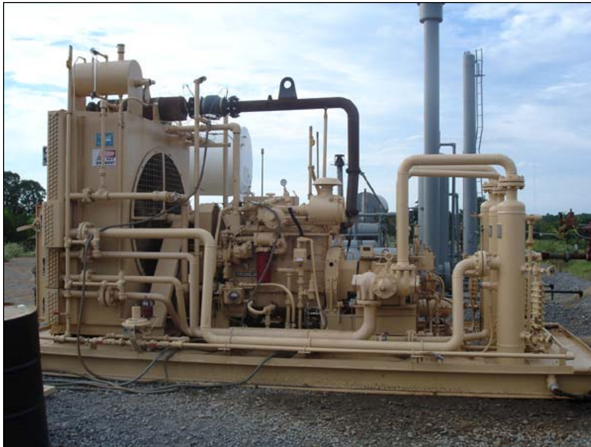
Figure 5-1. Retrofit system showing catalyst installation in compressor exhaust line.
